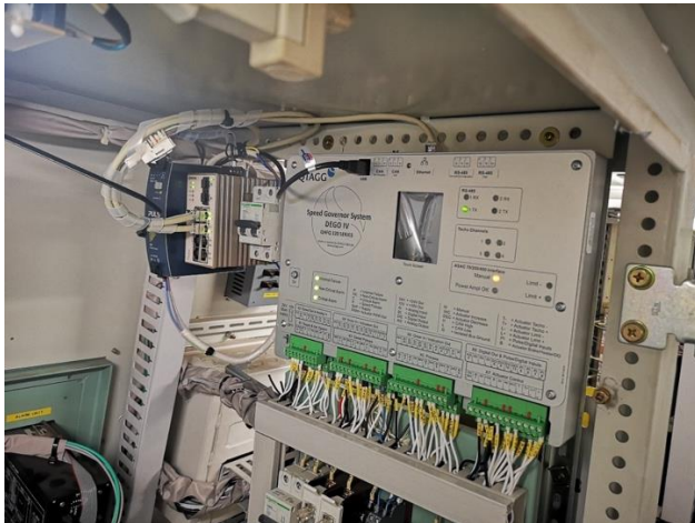
Westermo's Lynx switch installed next to Qtagg's DEGO speed governor system.
