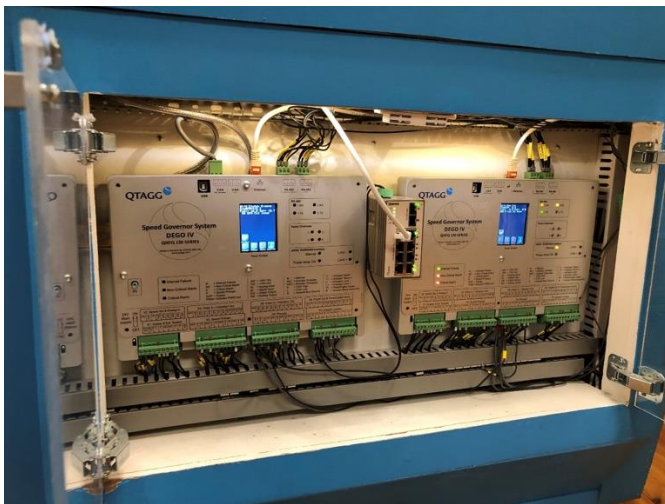
Westermo's Lynx switch installed on Qtagg's test rig
